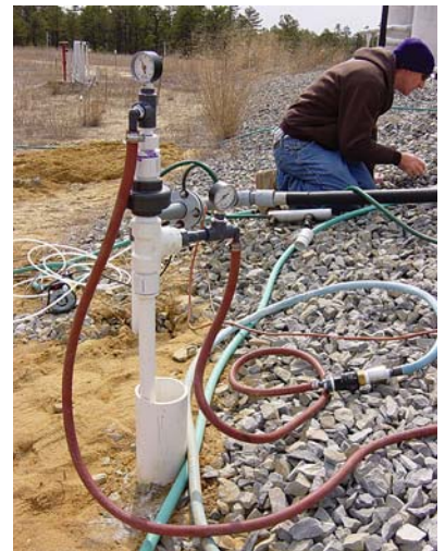
ADAS system well head
